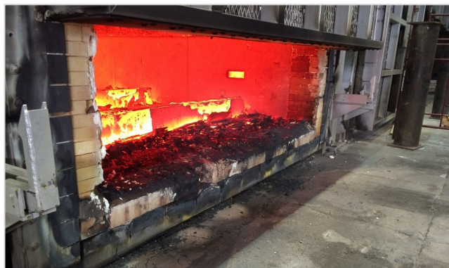
ARMORMAX® sill after 36 months in service
