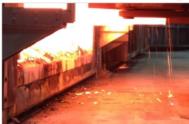
ARMORMAX® sill after 18 months in service
