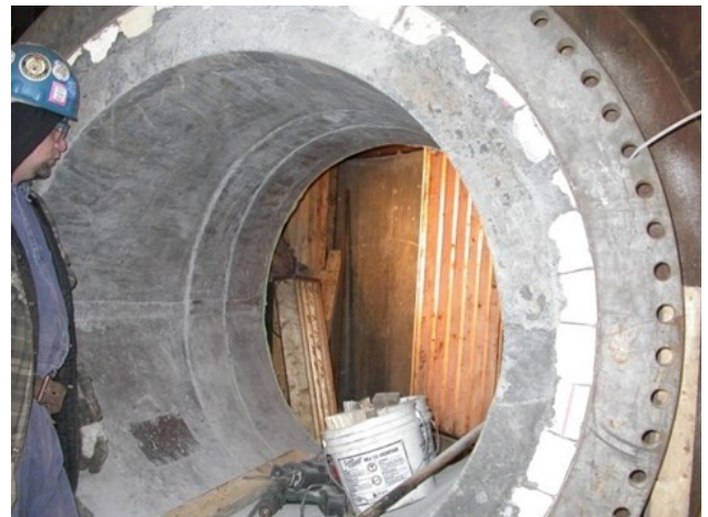
Cast hot blast outlet
