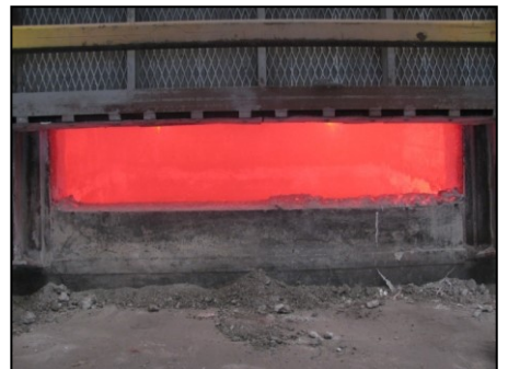
ARMORMAX 70 AC sill after 10 months of service
